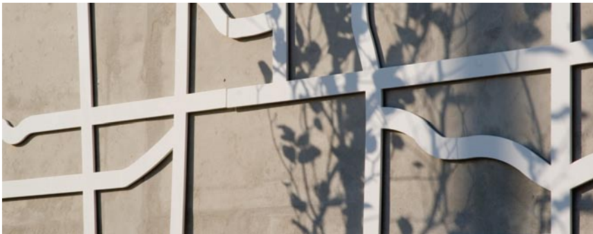
Detail of a portion of the Map Wall Artwork along the South elevation
